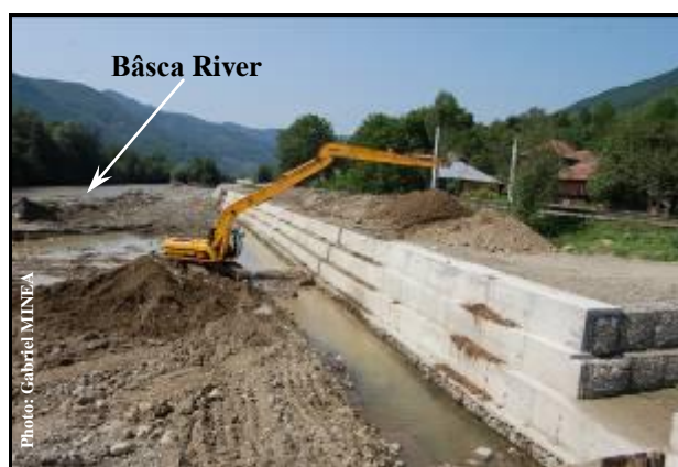
Photo 2 New hydrotechnical arrangements (gabion baskets) on the Bâsca River (august 10 th 2010)
