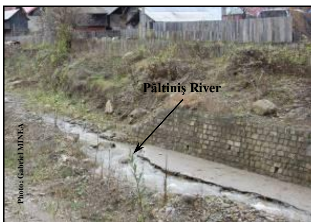
Photo 1 Hydrotechnical work destroyed by the flood from July 20 th 2002 (near the confluence of the Păltiniș with the Bâsca River)
